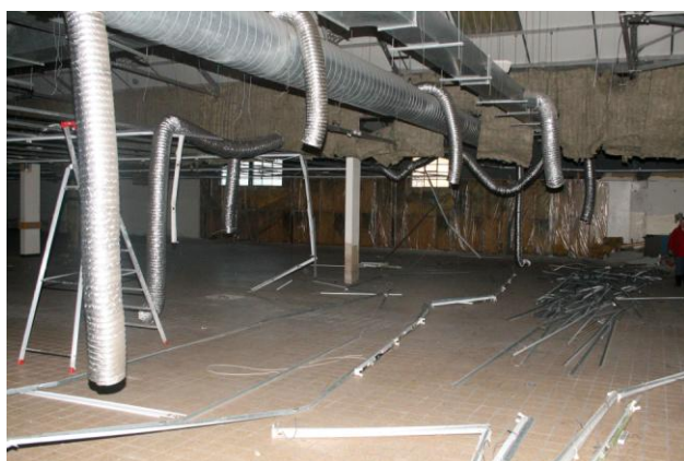
All the Way Up: The Open Roof Space with Heating Ducts
